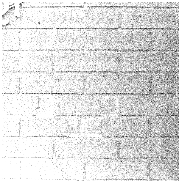
Brick Cladding fallen off wall
